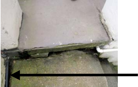
26: Check random pipe and remove or paint dark to show up on step
