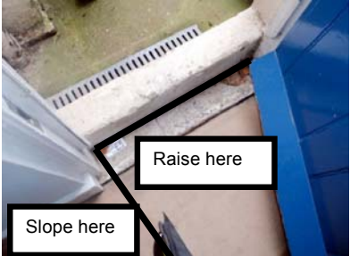
27 (a): If new flooring is installed, consider a slope or ramp down from the threshold or raise the flooring to the threshold
